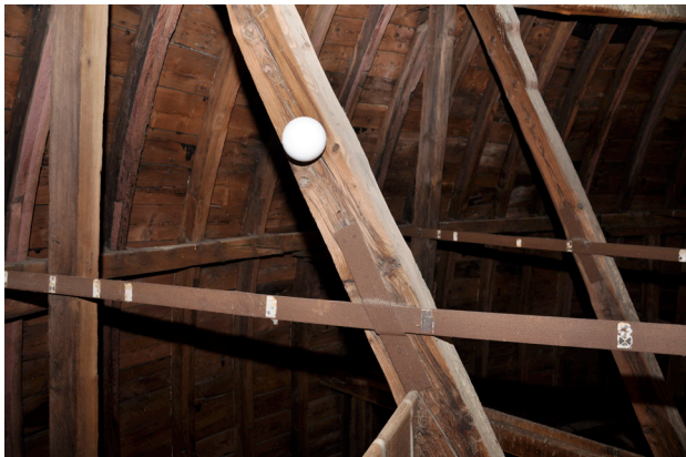
Figure 4. The wooden structure and one of the spherical target that we used for the survey.
