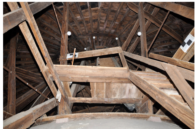
Figure 3. The wooden structure of the dome and of the staircase that takes people up to the top.
