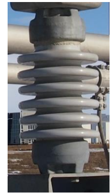
Figure 6. An insulator in the electrical substation
