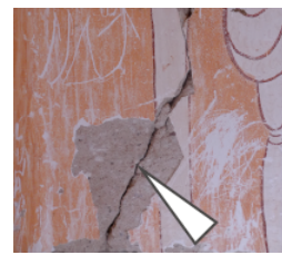
c. Structural cracking
