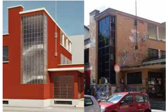
Figure 13. Comparison of digital reconstruction and current condition of the 'Casa rionale del Balilla di via Guastalla'. BIM model by G. Businaro.
