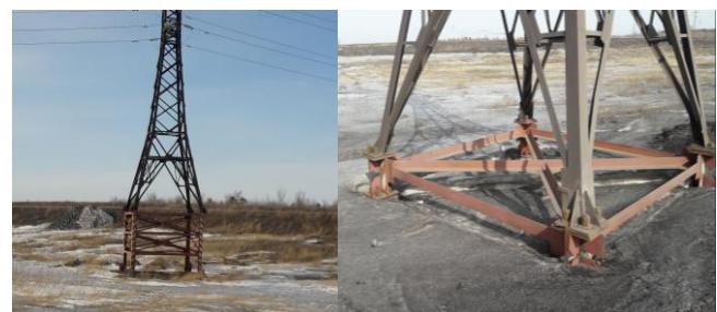
Figure 8. The reconstructed electric transmission lines, which are on the undermined territory of Kuzembayev mine.
