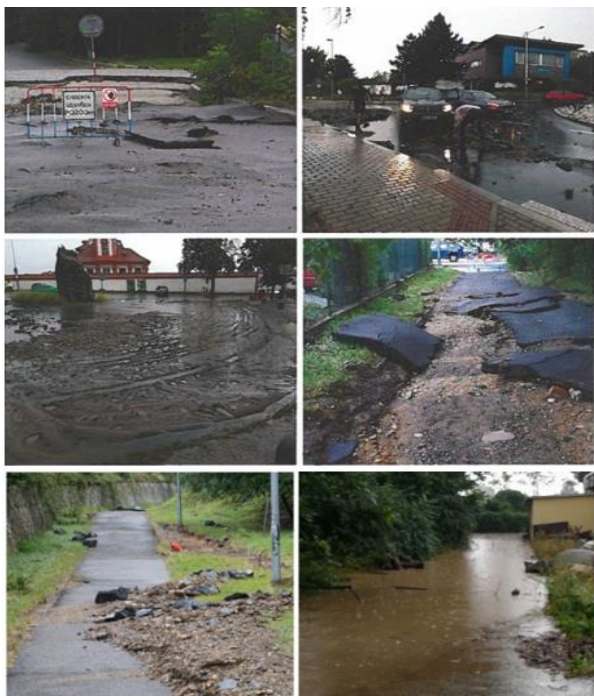
Figure 4. Photo documentation of cloudburst damage
