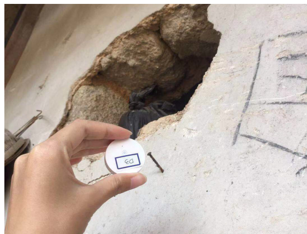
Figure 8. Humidity sensor used in Monitoring Dafudi
