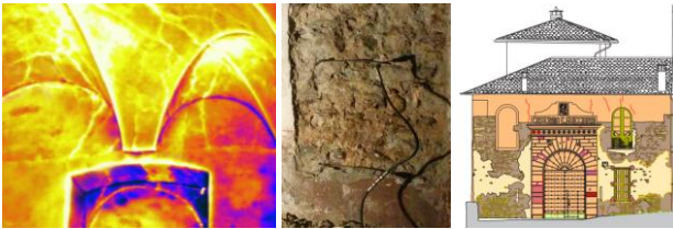
Figure 9. Thermographic image revealing hidden cracks in the vault, double flat-test, condition map with the identified degradations.
