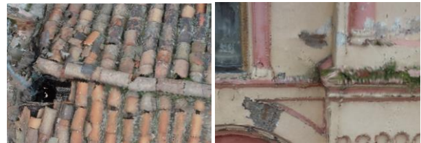
Figure 14. Damages in the church of Nabón
