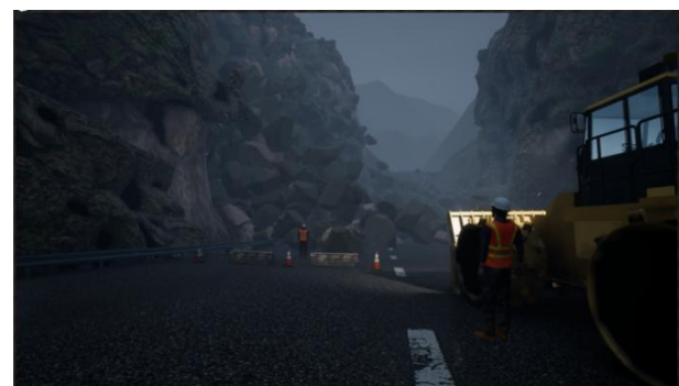
Figure 10. Block the road and clean up the scene of the accident
