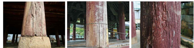
Crack Exfoliation Deterioration Figure 2. Major types of damage at Yeongnamnu Pavilion
