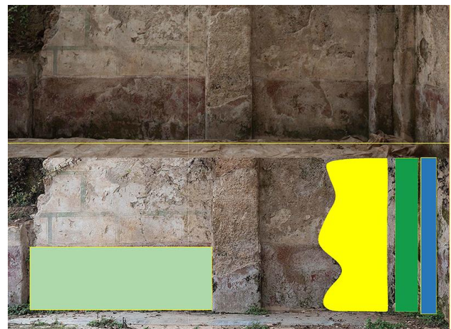
Figure 14. Comparison degradation surfaces in the surveys 2010-2019 of the external side wall
