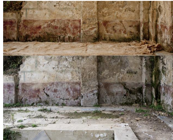
Figure 13. Visualization of degradation images, in the surveys 2010-2019, of the external side wall
