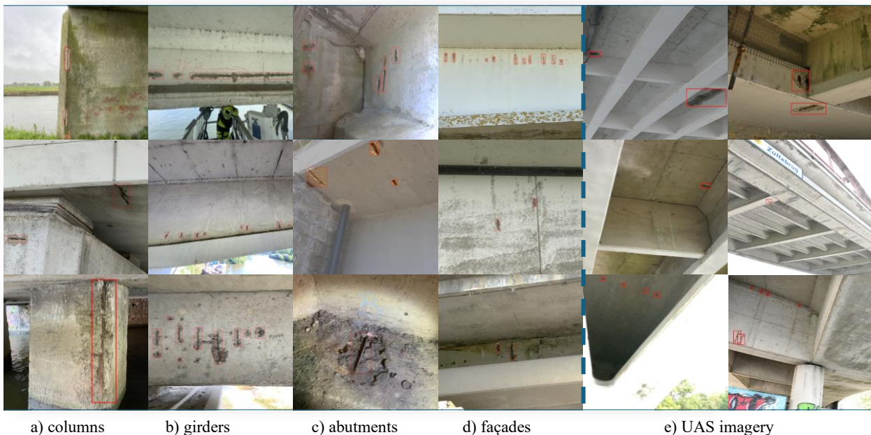
Figure 1: Variety of ER appearance and visual differences between documentation and UAS inspection images. ER appears in various forms and on various structural elements but are typically central and quasi-orthogonal (a-d) while UAS imagery contains damages in the background, typically smaller and in various lighting conditions (e).
